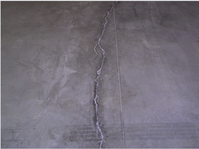
Crack in a newly laid carpark floor
