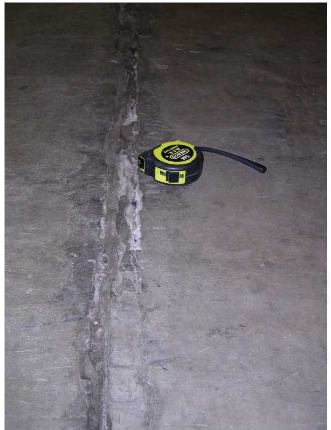
Damaged joint in need of repair
